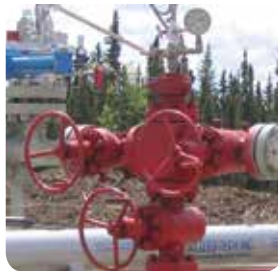
Wellhead Gate Valve
